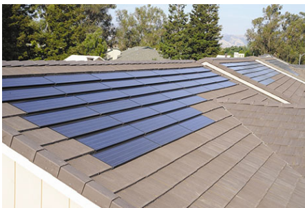
Integrated solar panels
