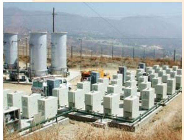
Figure 9.12 Landfill gas energy generation facility
